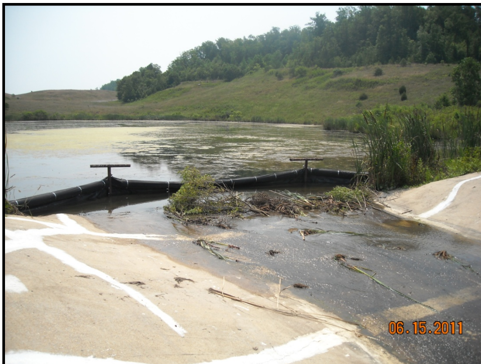
Photo B.247 – Treatment Pond Outfall DRMW-3 – Looking upstream – June 15, 2011
