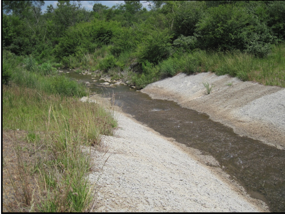
Photo B.218 – Treatment Pond Outfall BMWW-36 – Looking downstream – May 25, 2011
