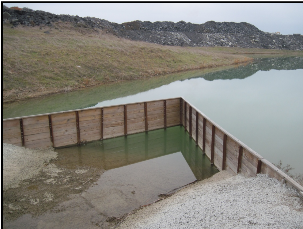
Photo B.209 – Treatment Pond Outfall BMWW-36 – Looking upstream – January 20, 2011
