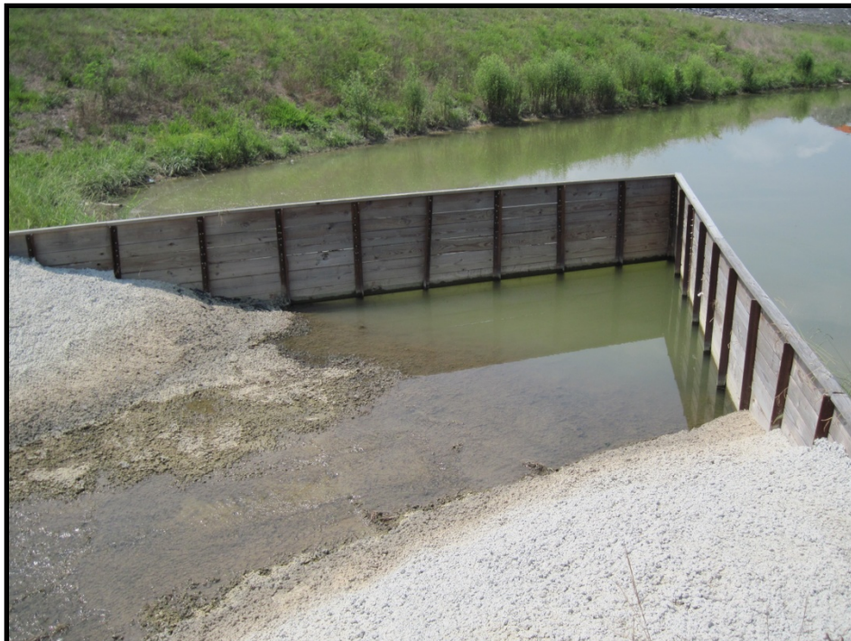
Photo B.221 – Treatment Pond Outfall BMWW-36 – Looking upstream – July 26, 2011
