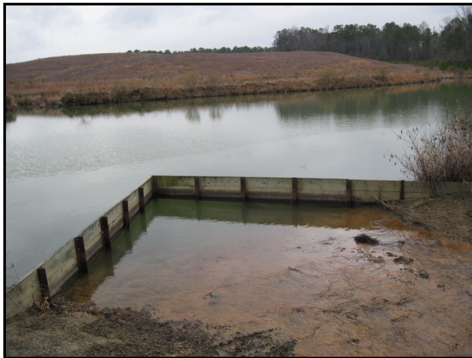
Photo B.189 – Treatment Pond Outfall BMWW-21 – Looking upstream – January 31, 2011
