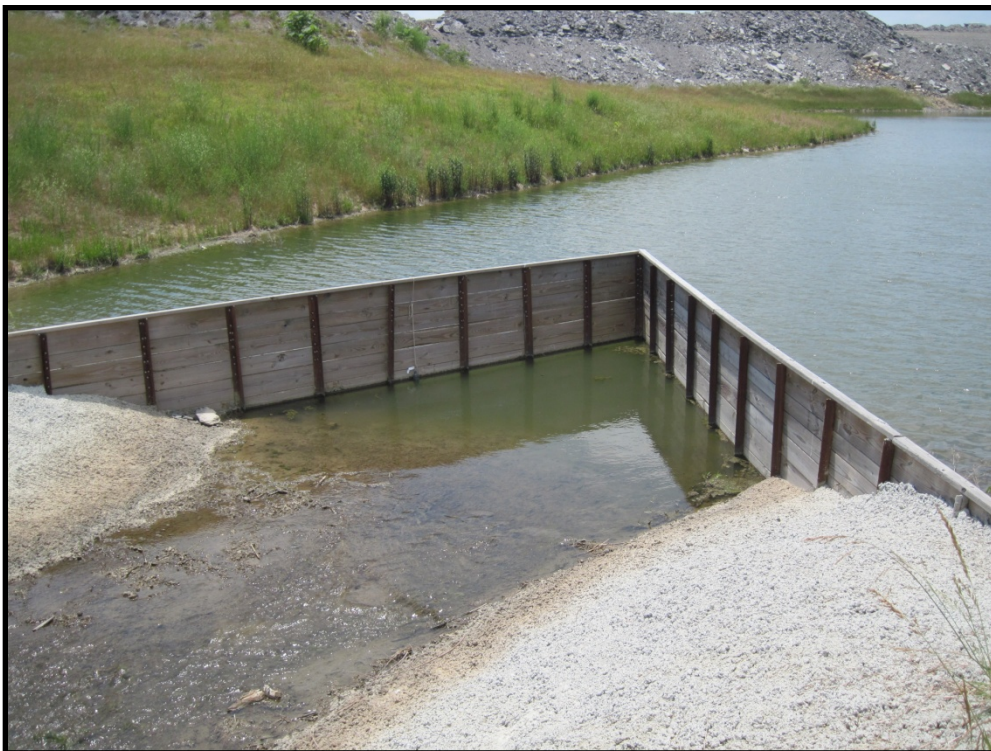
Photo B.217 – Treatment Pond Outfall BMWW-36 – Looking upstream – May 25, 2011
