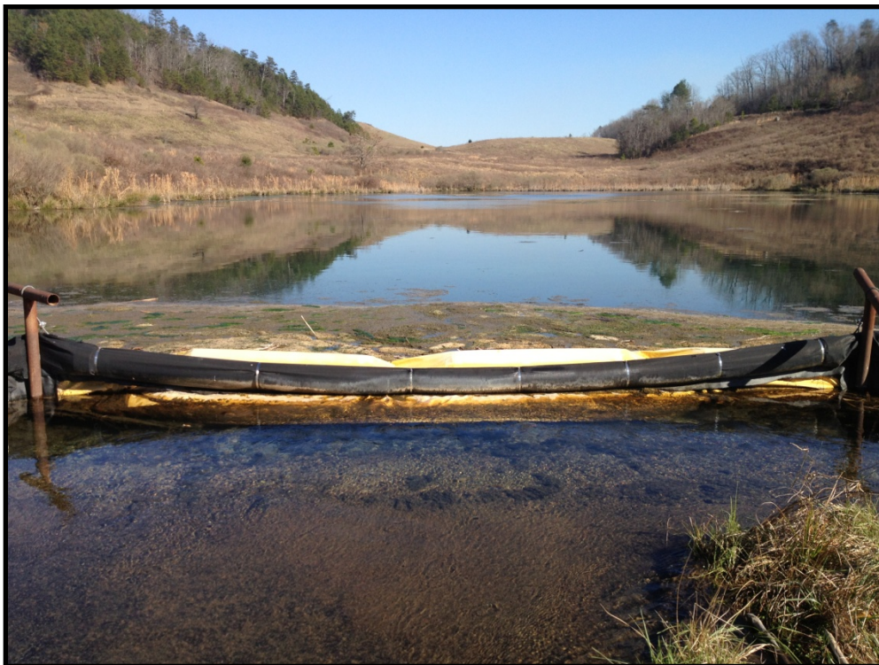
Photo B.253 – Treatment Pond Outfall DRMW-3 – Looking upstream – January 22, 2013
