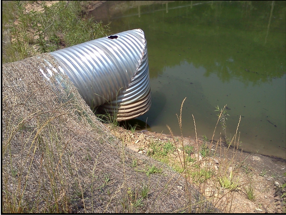
Photo B.276 – Treatment Pond Outfall WIMJ-1 – Looking upstream – June 9, 2011
