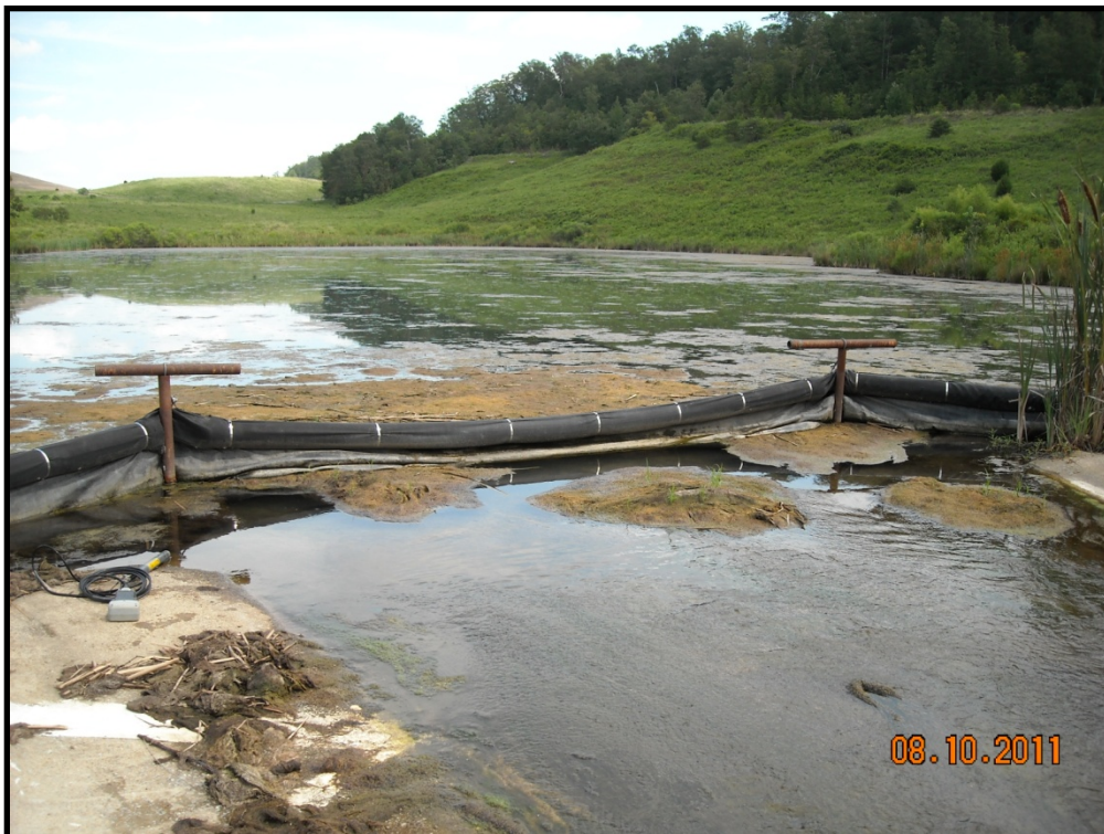
Photo B.249 – Treatment Pond Outfall DRMW-3 – Looking upstream – August 10, 2011
