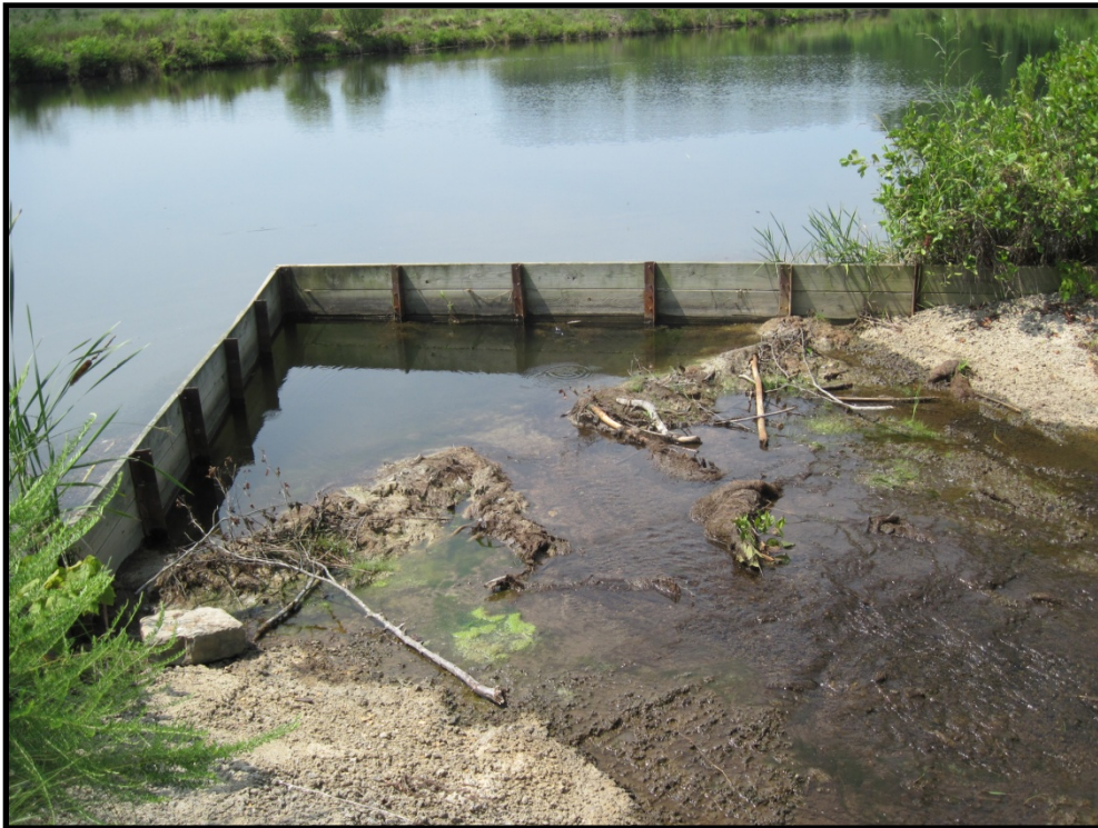
Photo B.201 – Treatment Pond Outfall BMWW-21 – Looking upstream – July 11, 2011
