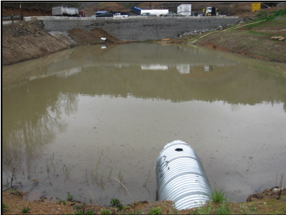
Photo B.273 – Treatment Pond Outfall WIMJ-1 – Looking upstream – March 31, 2011
