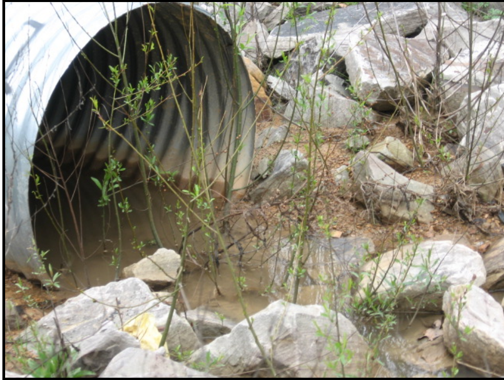
Photo B.274 – Treatment Pond Outfall WIMJ-1 – Drainage from pond – March 31, 2011
