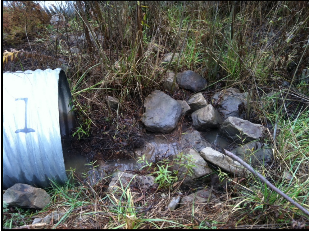
Photo B.278 – Treatment Pond Outfall WIMJ-1 – Discharge from pond – December 5, 2012
