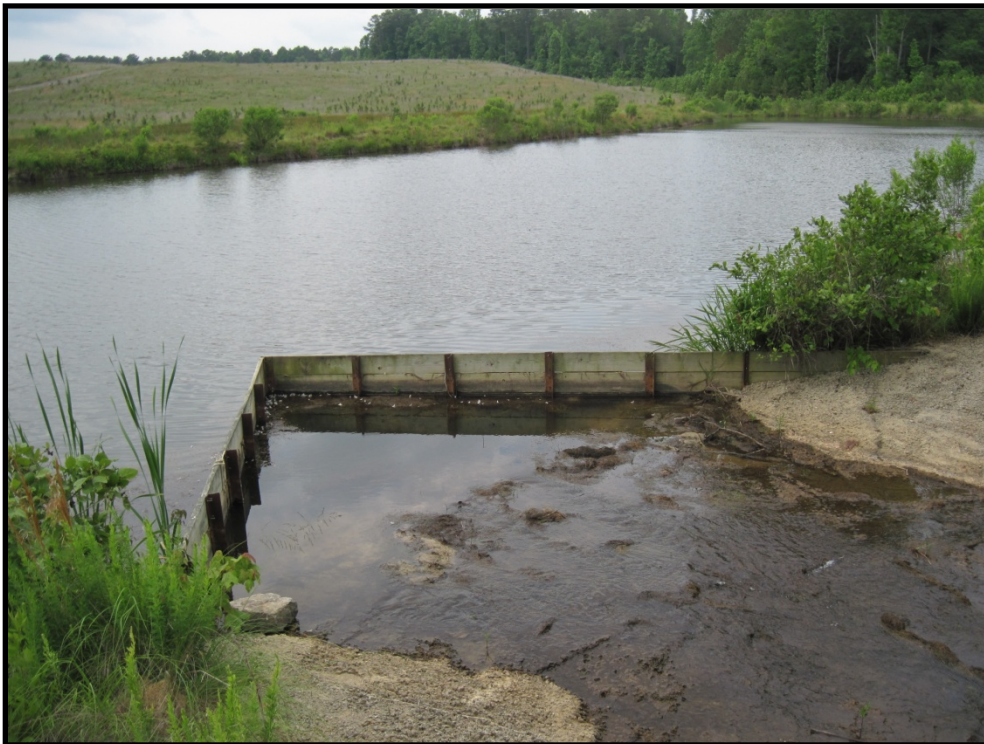
Photo B.197 – Treatment Pond Outfall BMWW-21 – Looking upstream – May 24, 2011
