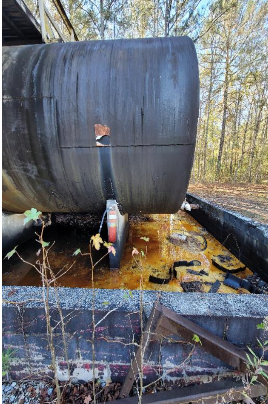
Approximately 2 inches of yellowish-orange oil/petroleum/cleaning fluids accumulating
