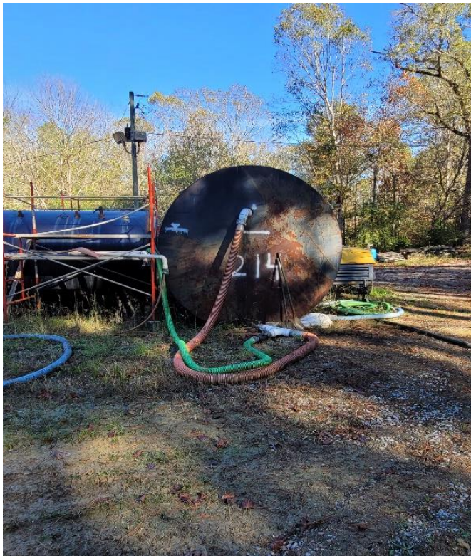
2 horizontal tanks placed directly on the ground in the area between the access road and tank area
