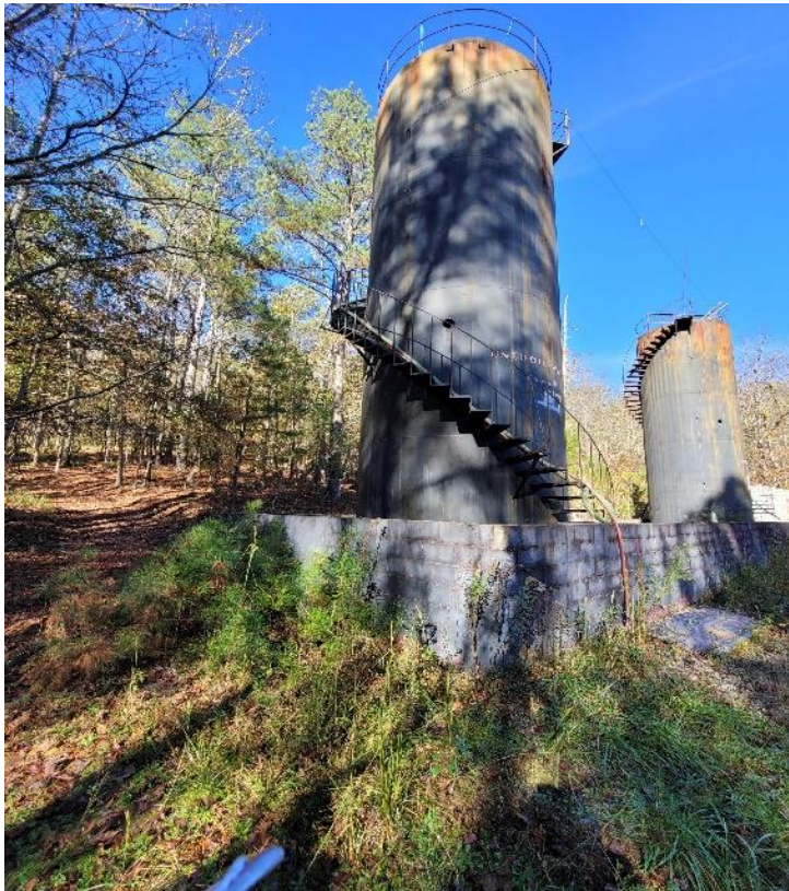
Vertical tanks with secondary containment area #2
