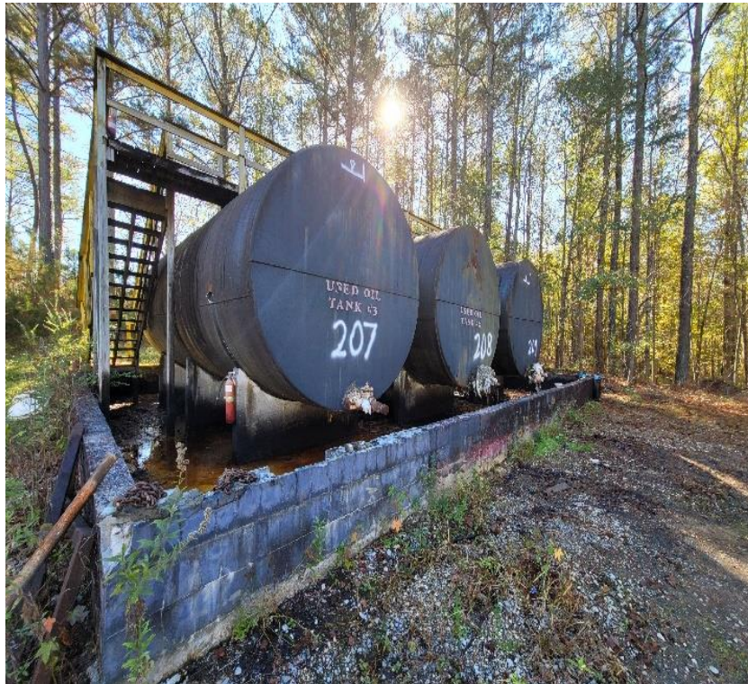
Horizontal tanks with secondary containment area #1
