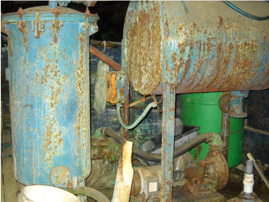
Transformer and equipment, A-1 Plating
