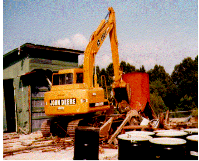
Initial excavation and removal efforts at Fulco Lumber Company, Haleyville, Marion County
