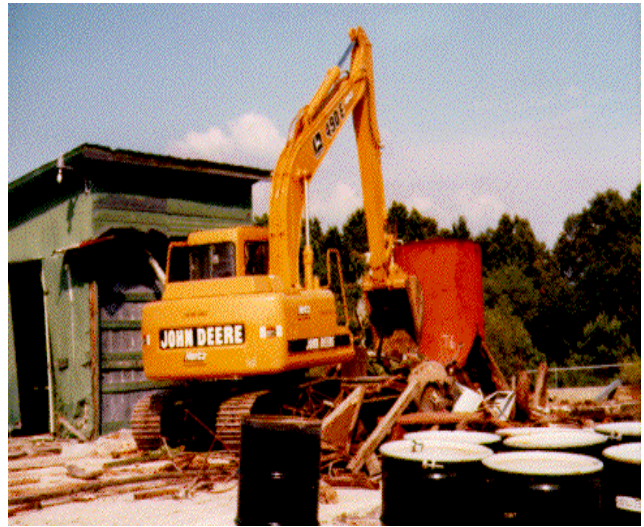
Initial excavation and removal efforts at Fullco Lumber Company, Haleyville, Marion County
