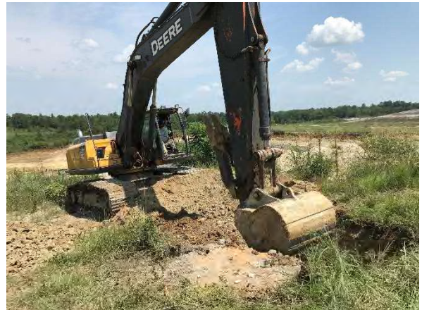
Photo #26 Excavating immediately adjacent to outer well casing to locate broken inner well casing.
