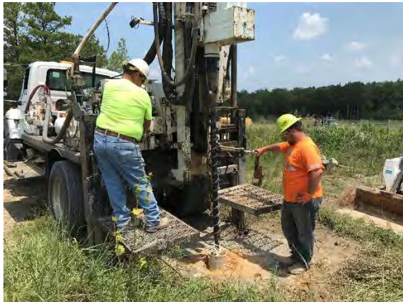
Photo #25 Overdrilling of BG-1 before inner well casing broke about ten feet below grade.
