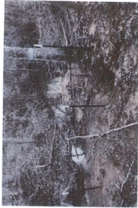
Upstream of low water stream crossing at 14.307470. RS 01214. Stream banks did not appear to have adequate protection.
