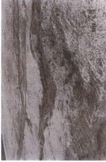
Emergency spillway of dam Slopes did not appear to be properly stabilized Erosion rills and gullies observed on site
