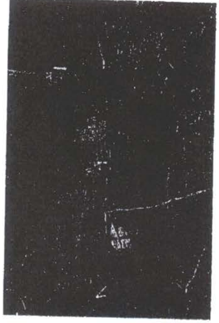
-Upstream of low water stream crossing at 33.007470 -85.317142. -Stream banks did not appear to have adequate protection.
