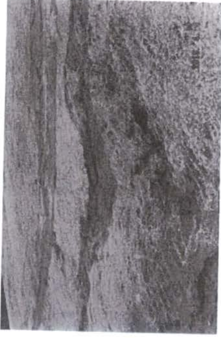
Emergency spillway of dam slopes did not appear to be properly stabilized. Erosion rills and gullies observed on site.
