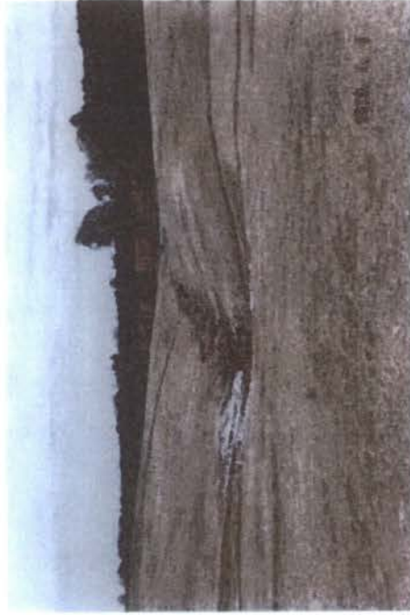
View facing northeast from dam of impoundment Slopes did not appear to be properly stabilized Erosion rills and gullies observed on site
