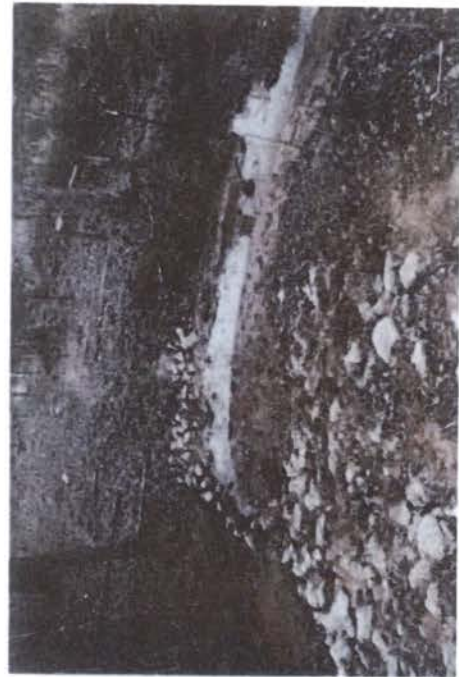
Low water stream crossing at 14.307470. RS 01214. Stream crossing does not appear to be adequately stabilized.
