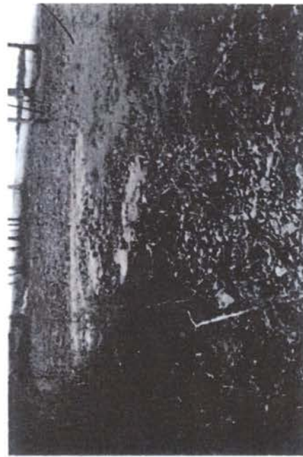
Sediment observed leaving the site and is being deposited on adjacent property.
