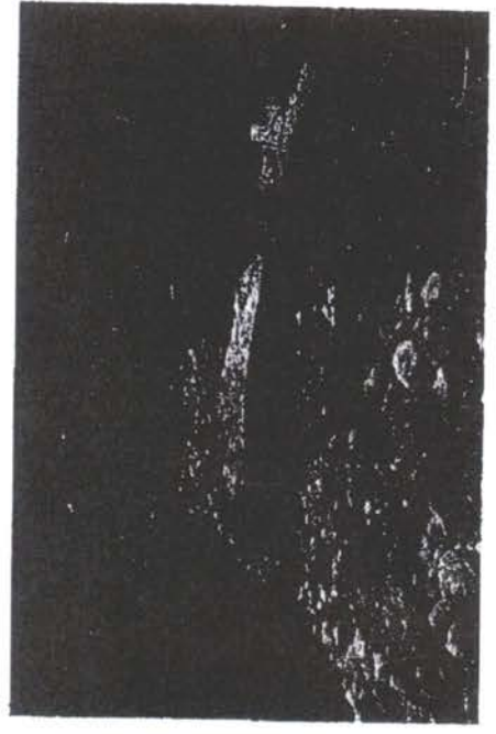
-Low water stream crossing at 33.007470 -85.317142. -Stream crossing does not appear to be adequately stabilized.
