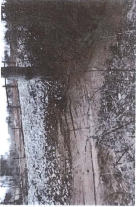
Stream crossing at 44.006546, 85.419871. Sediment observed leaving the site and is being deposited on adjacent property. Sediment observed leaving the site and entering an unnamed tributary to Veasey Creek.
