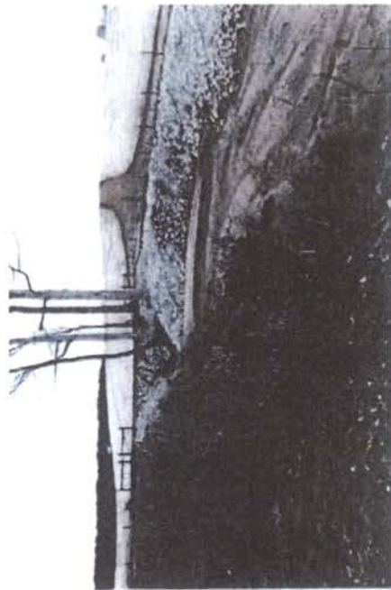
Sediment observed leaving the site and is being deposited on adjacent property.
